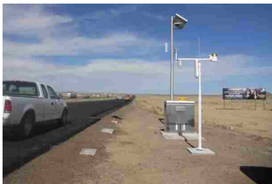
Figure 23. Installed weather station
